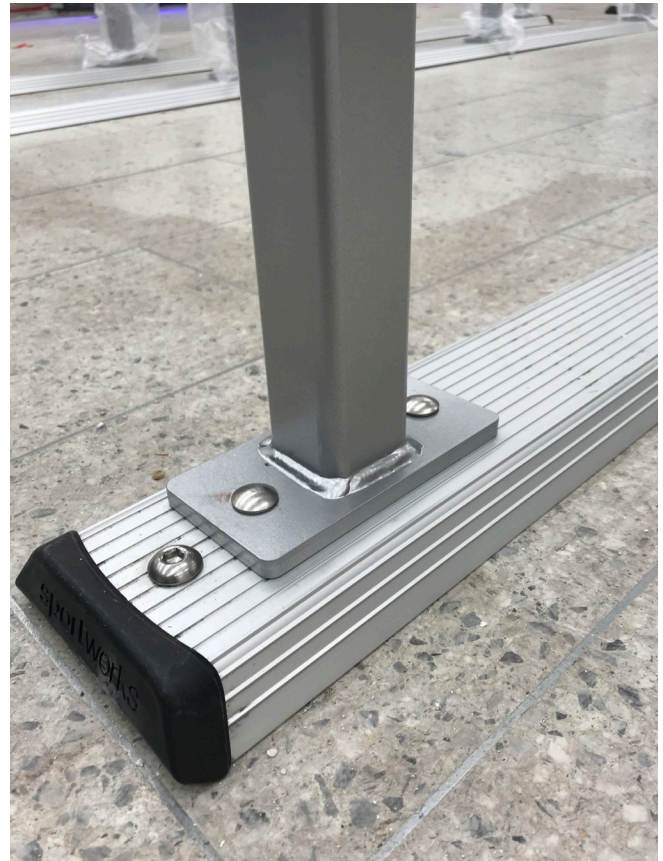
Bolt-on aluminum channel rail-mounted racks anchored to terrazzo floor, 19th Street BART Station, Oakland CA (Photo: Heath Maddox)
